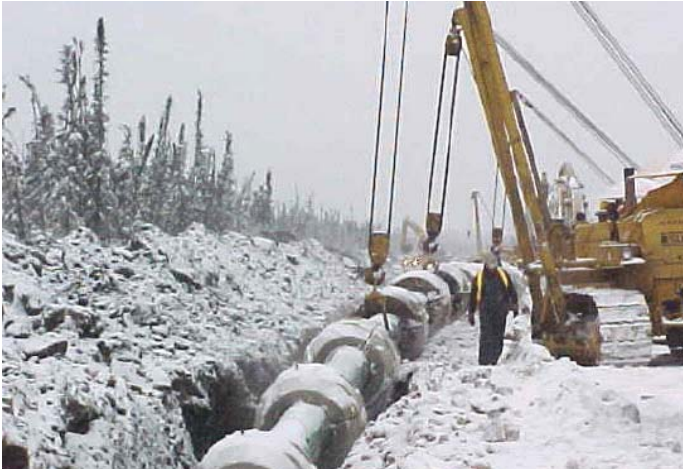
Figure 6: An NPS 24 Bolt-on Weighted Section of Pipe is Lowered into the Ditch
